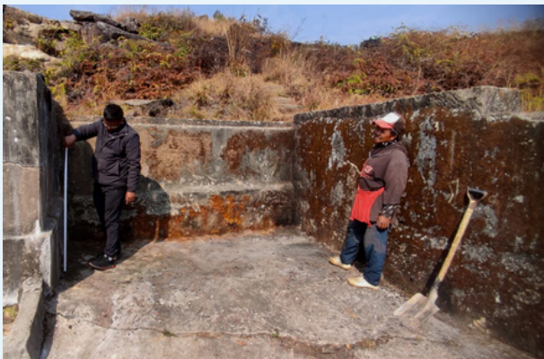
Site instruction for operation of open limestone channel (OLC) at Laitryngew, Shella block under MLAMP.
