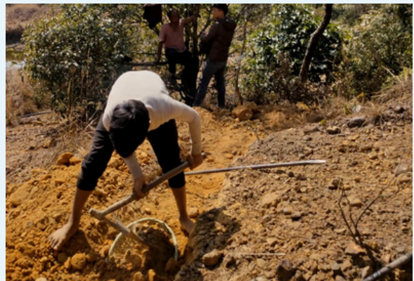
Site instruction for on-going open limestone channel (OLC) work at Laitmawsiang, Laitkroh block under MLAMP.
