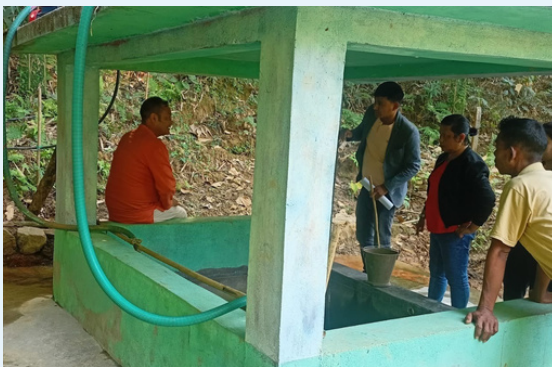
Inspection of spring chamber at Muji Agalgre village with SWGH, DC and DPMU staff.
