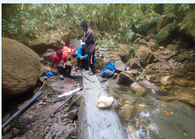
Site visit for construction supervision of checkdam, penstock laying and alignment at Domtynrong village, Mawkyrwat Block, South West Khasi Hills district.
