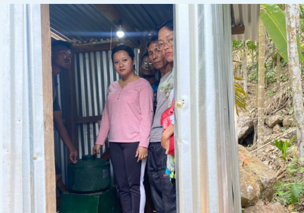
Successful installation of Hydroger at Dengasi Village Rerapara Block, South West Garo Hills district.
