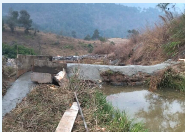
Site visit for supervision of construction of checkdam at Mawpdang village, Mawryngkneng Block, East Khasi Hills district.
