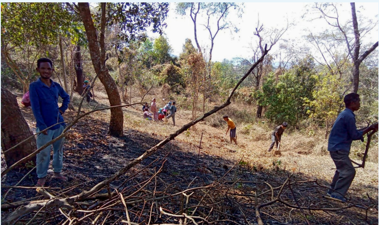
Preparation of land for construction of Community Hall at Chandigre under Rongram land
