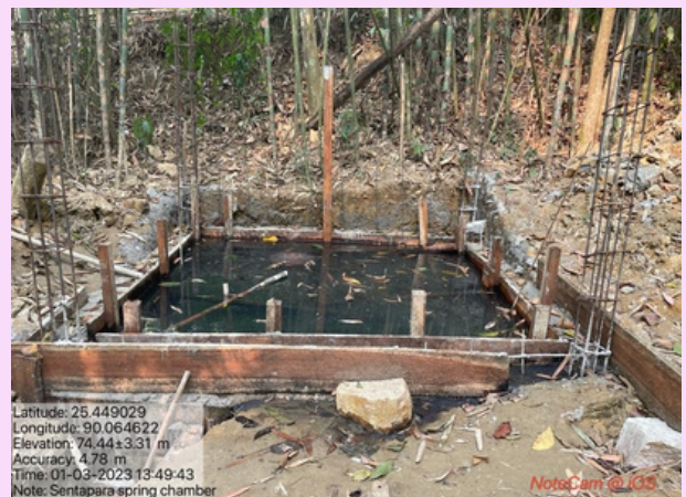
Field visit for the inspection of spring chamber by Field Engineer (EE)
