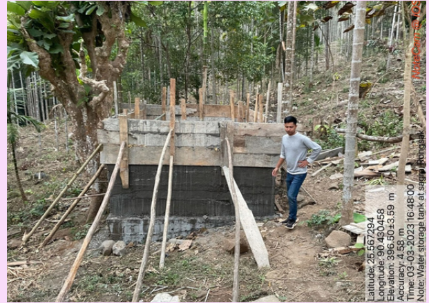
Site inspection on RCC dam and Water storage tank under catalytic fund
