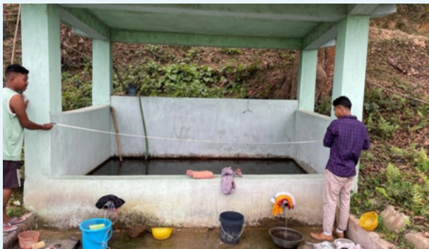
The Field Engineer visited Sonabil village to take measurements for the installation of a safe gate for the spring chamber
