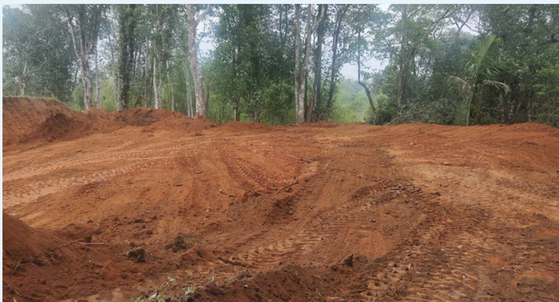
Kalak Songgital, Samanda Block, EGH, has started preparing land for Community Hall
