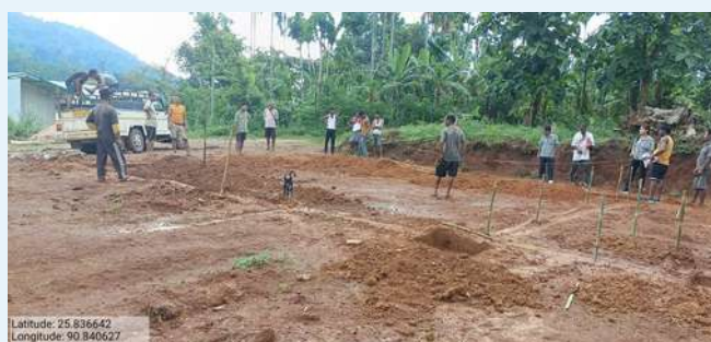
Earth work foundation in progress for Community Hall at Lower jambal Village under Kharkutta C&RD Block.
