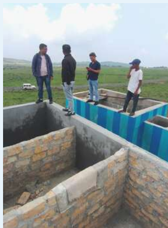
Site inspection to Laitmawsiang and Laitduh village under Laitkroh Block, East Khasi Hills district.
