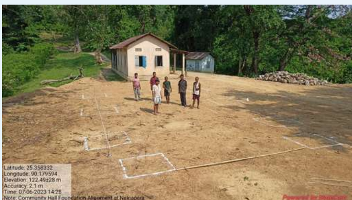
Column alignment done for CH by FEs at Nalnapara Village, Gambegre Block.
