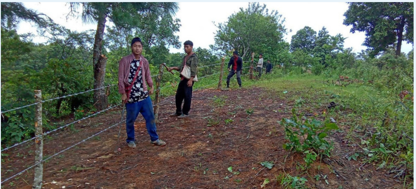
Fencing on private land was successfully completed at Buangkhor Mual village on August 22, 2023.
