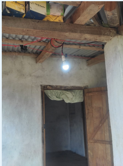
Site verification and electrification works at Saiden village under Umling block and Lamalong village, under Umsning block Ri-Bhoi district.
